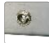
10mm press studs for earth bonding.
